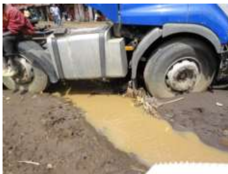
(a) Drainage problems
