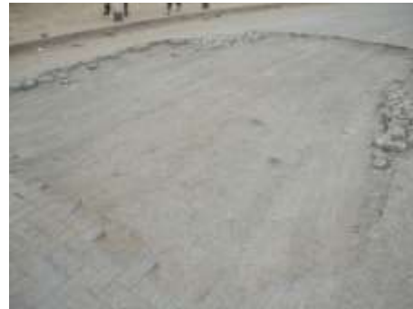
(b) The deteriorating state of the parking
